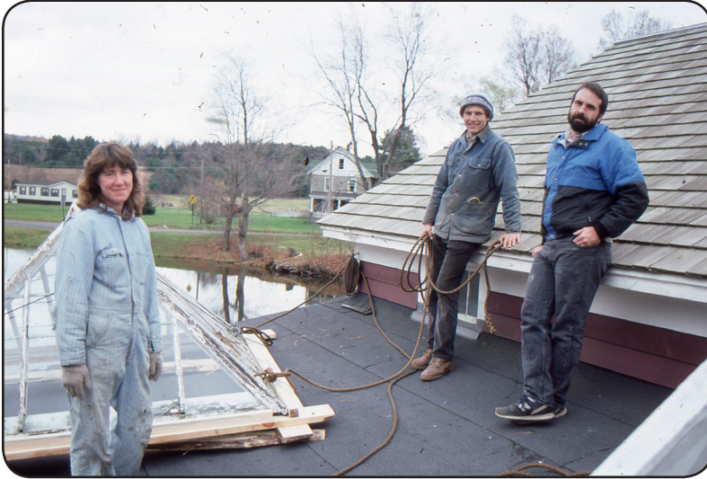
Dawn with Steve Eastman and Keith Bott working on the skylight above the box room in 1988
