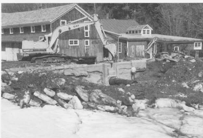
In 1993, we could use a backhoe to remove dirt from around the dam and to install the new flume pipe. The work was begun during the Winter, so the project would be completed by Spring. The museum hopes to have the pond dredged before its May opening in 2003.
